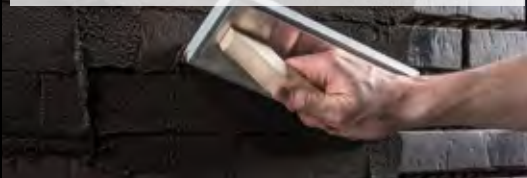
With the slurry method, the joints are filled diagonally with the grouting or plaster float. Walls should be worked from top to bottom.
