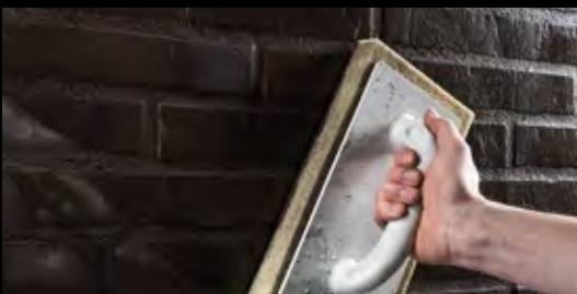
The excess grout is washed off diagonally using a plaster float with a sponge or foam pad.
