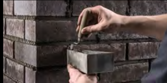
The vertical joints can be finished more easily with a smaller pointing trowel.
