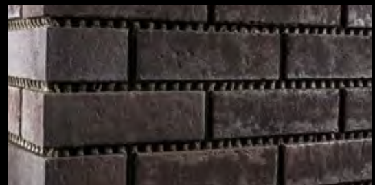
The finished surface. Grouting can be done after the appropriate drying time.
