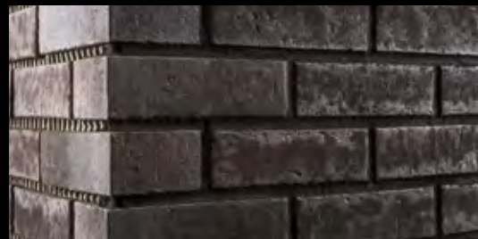
The finished joint pattern. Full masonry stretches are grouted at one go.
