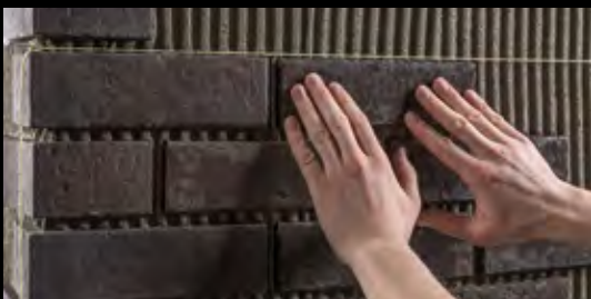
Use a string to plumb the clinker area. The clinker slips are pressed into the adhesive bed.
